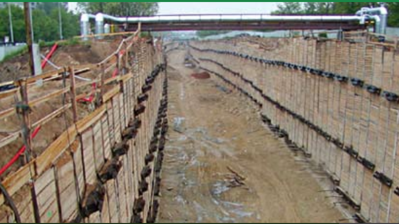
Open pit for the cut-and-cover tunnels between the Střížkov and Prosek stations
